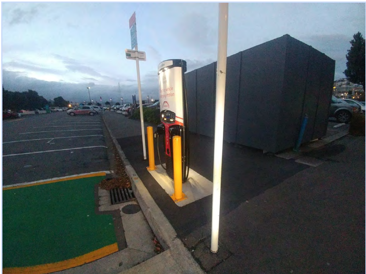
Electric car charging station. Wellington, New Zealand.
